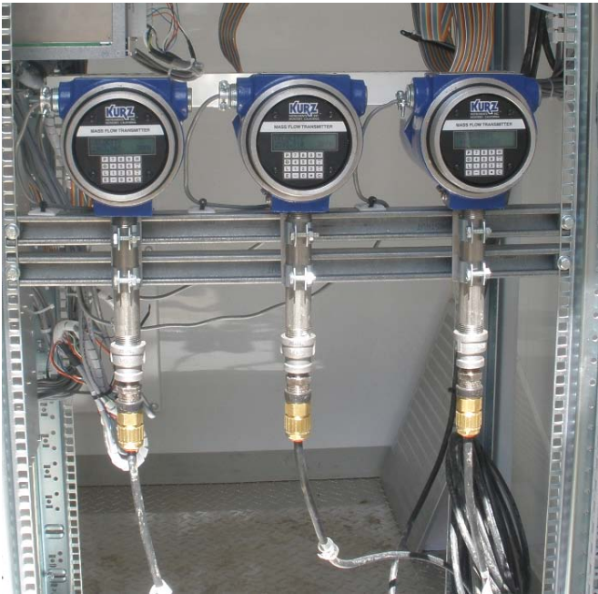
Cable Gland Example with Braided Shielded cable on a TS configuration.
